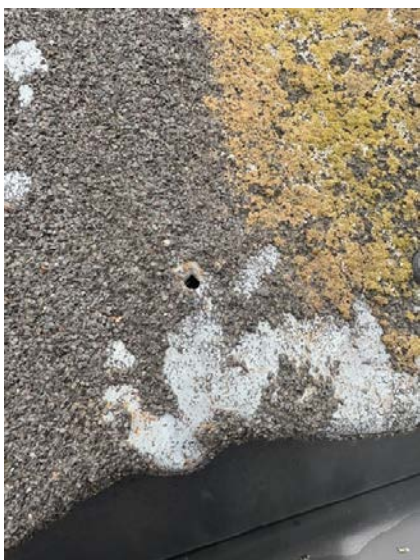
Hull i takteking.
