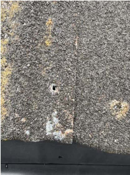
Hull i takteking.
