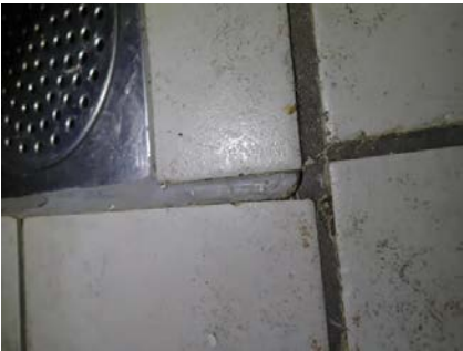
Riss i flisfuger.
