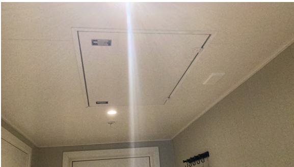
Aggregat i himling i gang.
