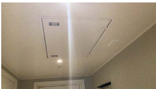
Aggregat i himling i gang.
