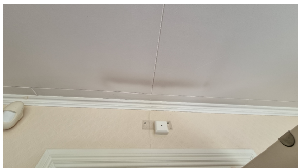
Misfarging i himling.
