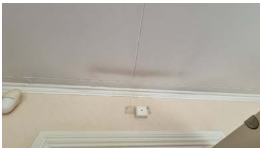
Misfarging i himling.
