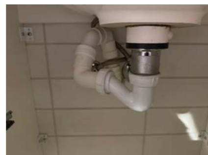
Røropplegg under servant.
