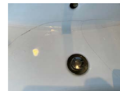
Sprekker i servanten
