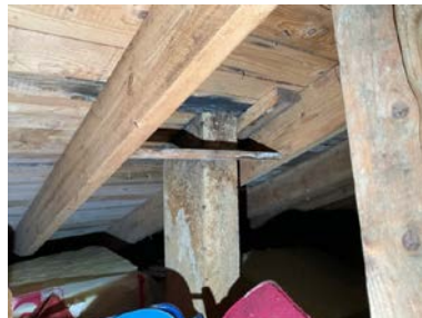
Fuktmerker i undertaket.
