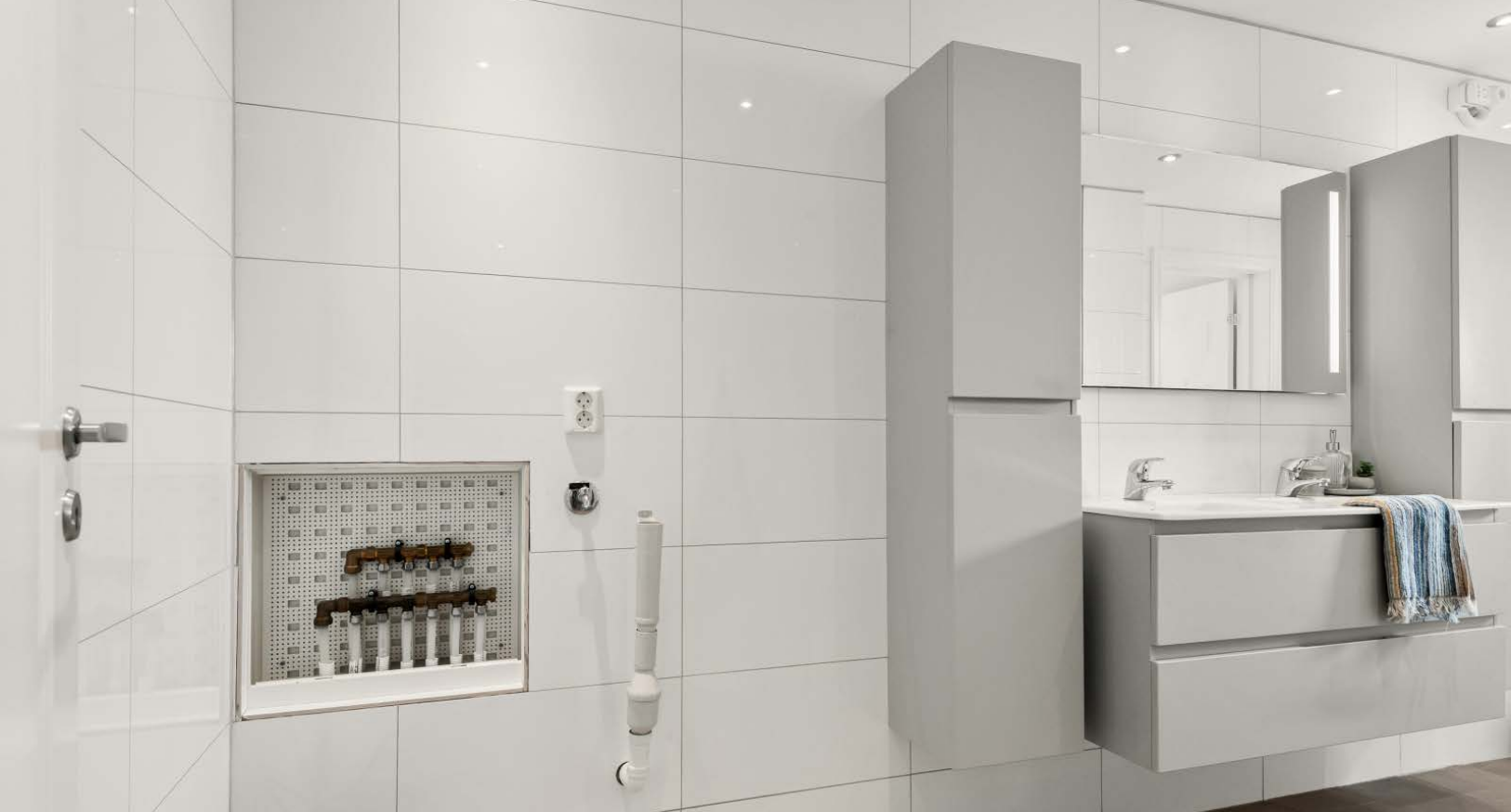
Opplegg for vaskemaskin.
