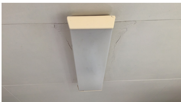
Folieslipp i himling.
