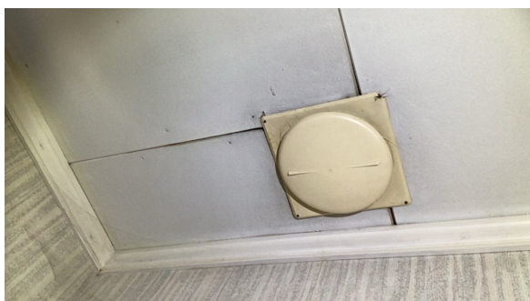
Fuktmerker i himling.
