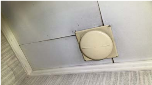
Fuktmerke i himling.
