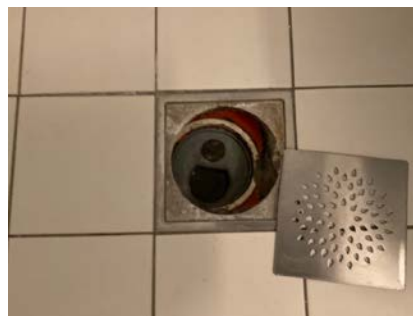
Plastsluk, eldre belegg
