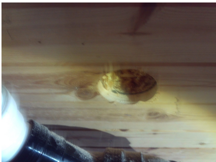
Hulltaking i underliggende himling.
