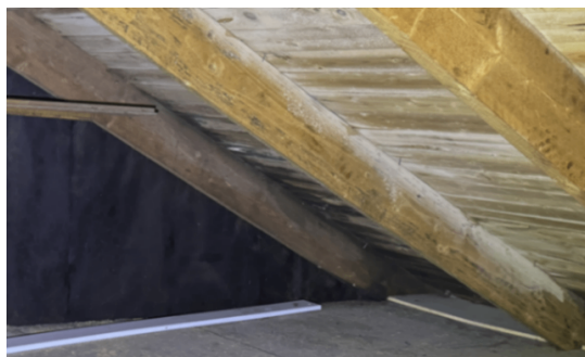
Fukt i undertak
