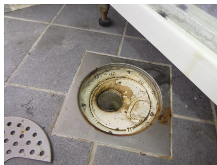
Sluk under kabinett
