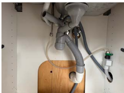
Røropplegg under vask.
