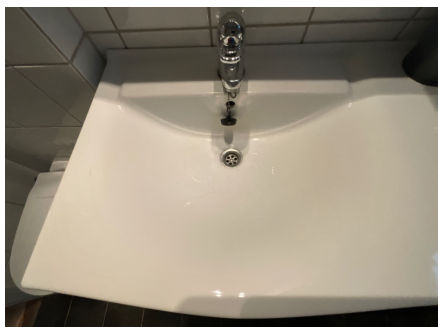
Krakelering i porselenet.
