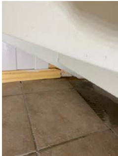
Manglende gulvflis, under trapp.
