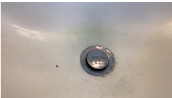
Riss i overflate i vask.
