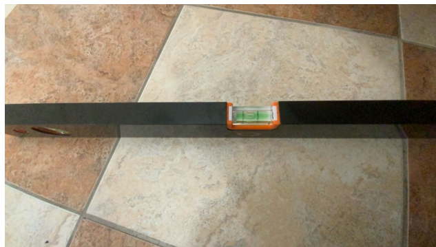
Litt motfall under vask.
