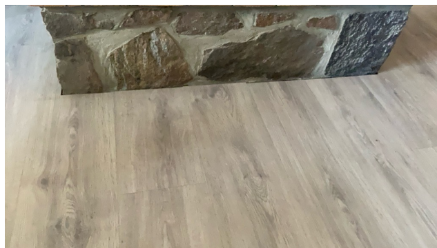
Ildfast plate mangler under/foran ildsted.
