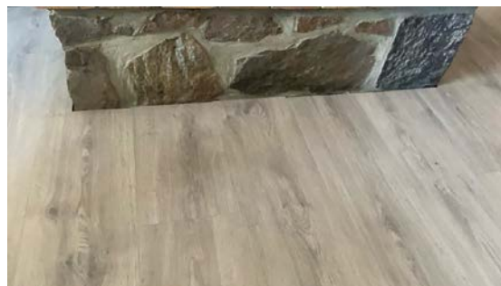
Ildfast plate mangler under/foran ildsted.
