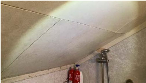
Fuktskader i himling.
