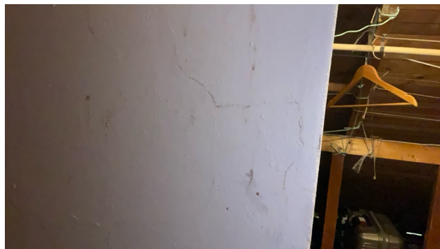
Riss/sprekker i pipe.
