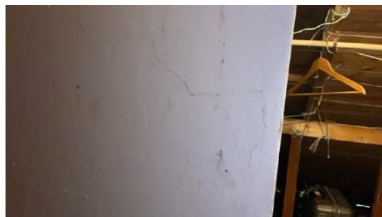
Riss/sprekker i pipe.
