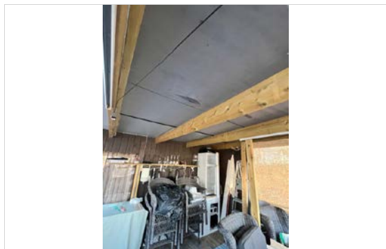
Fukt i undertak
