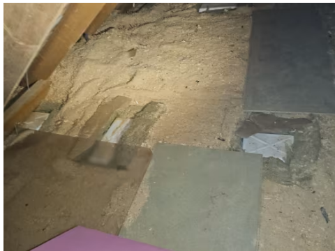
Mangelfull isolering over downlightkasser.
