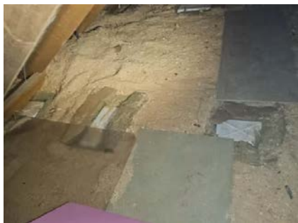
Mangelfull isolering over downlighstkasser.
