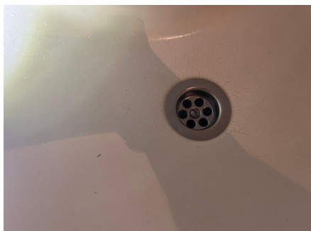
Sprekker/krakelering i servant
