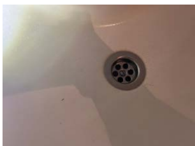
Sprekker/krakelering i servant
