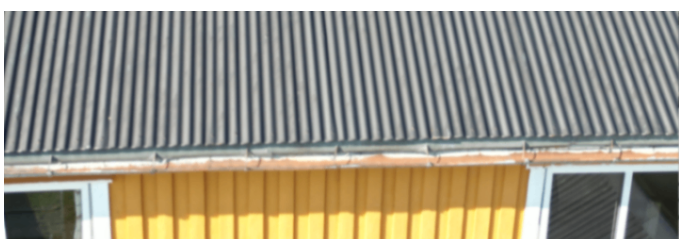
Rust i takrenner.
