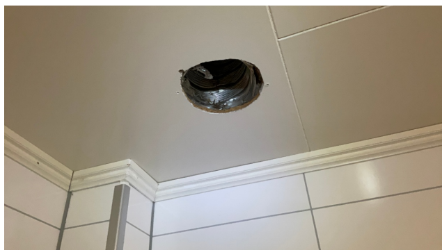
Manglende ventilrist for ventilering.
