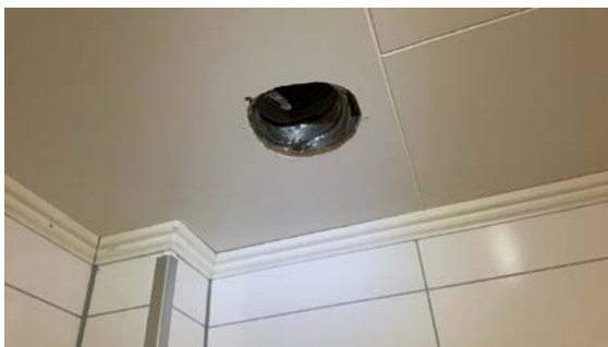
Manglende ventilrist for ventilering.
