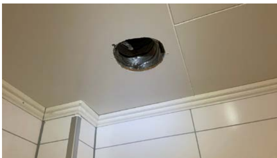
Manglende ventilrist for ventilering.
