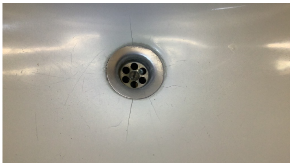
Riss i servant.
