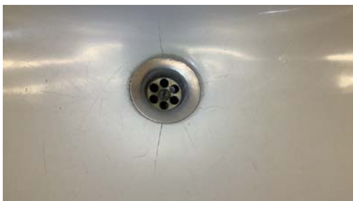
Riss i servant.
