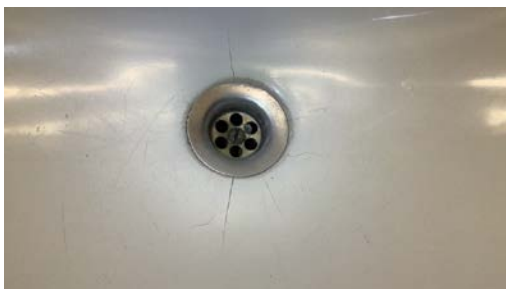
Riss i servant.
