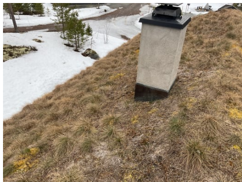
Manglende stige for feiing
