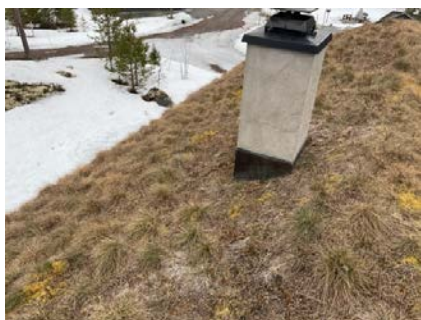
Manglende stige for feiing
