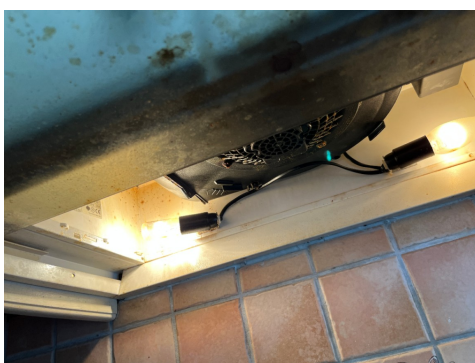
Manglende filter i ventilator
