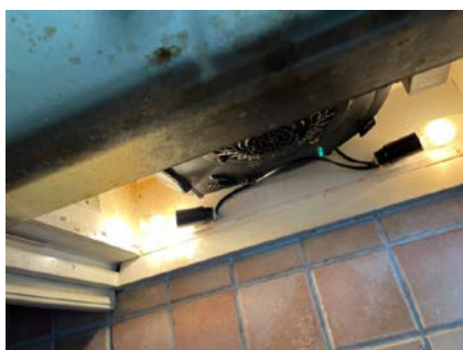
Manglende filter i ventilator
