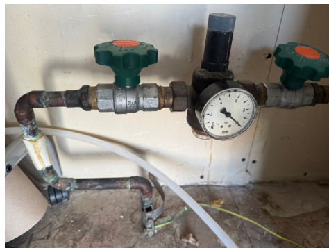
Stoppekran i bod.
