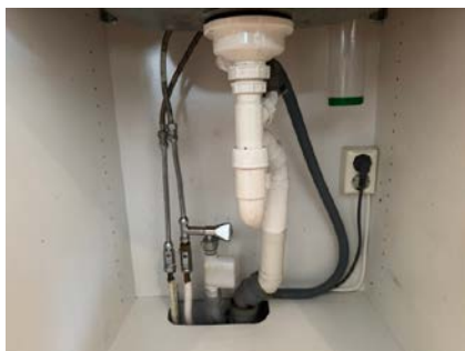
Røropplegg under vask.
