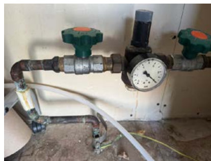
Stoppekrane i bod.
