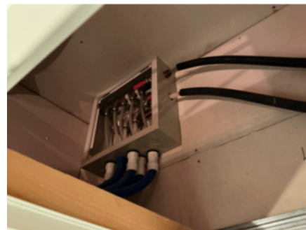
Fordelerskap over himling.
