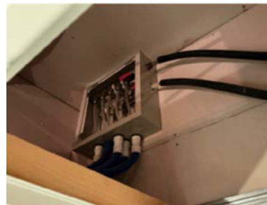
Fordelerskap over himling.
