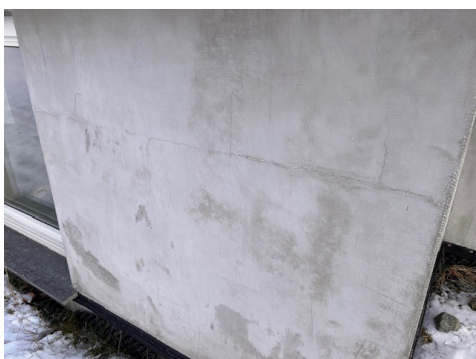
Sprekker i puss.
