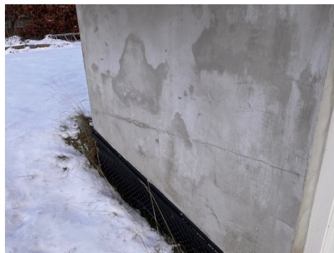
Sprekker i puss.
