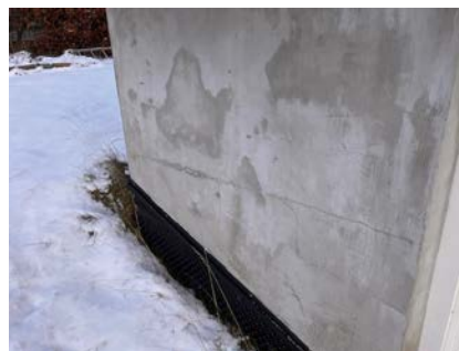
Sprekker i puss.
