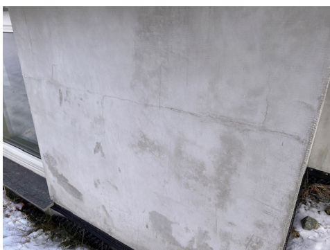
Sprekker i puss.
