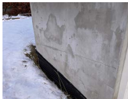
Sprekker i puss.
