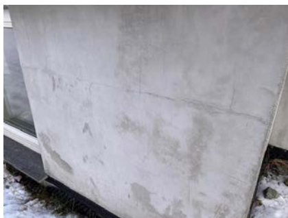
Sprekker i puss.
